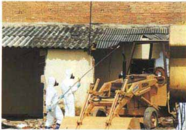
8. Monitoring the roof of the house of E.F.2 and S.F.1 during demolition.
