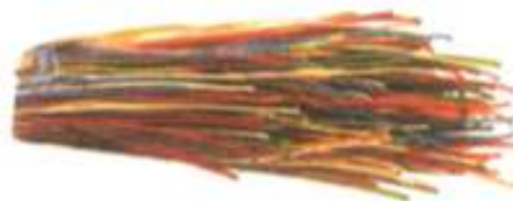
Cable with No Covering
